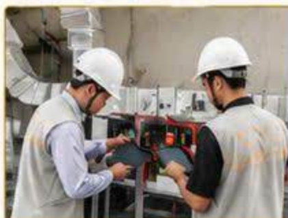
TESTING &amp; COMMISSIONING
